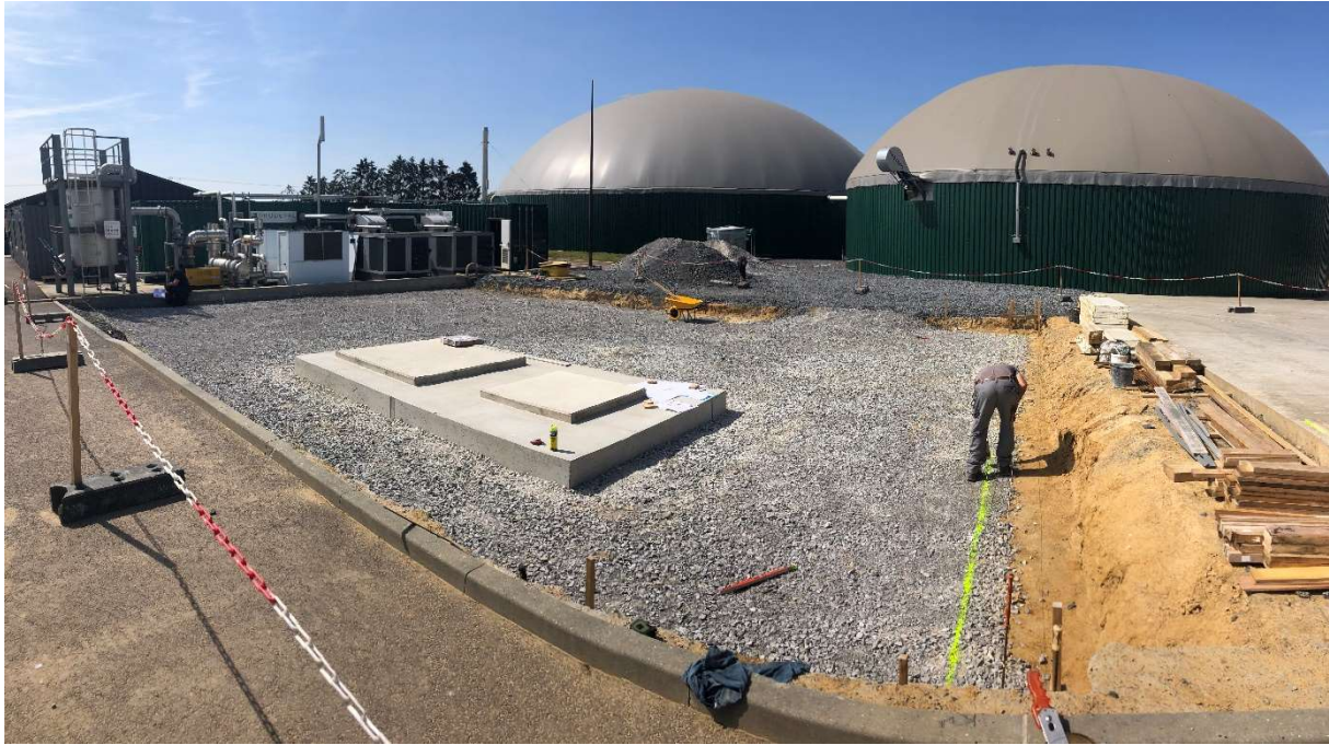
Construction work on the Enosis biological methanation installation coupled with the Energia Thiérache agricultural methanation unit – Photo credit:© Enosis.
